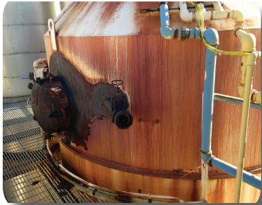
A severely corroded and unsafe combustion chamber
